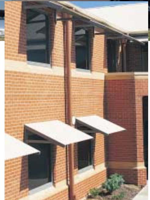
Bands of cream bricks envelop the building at the sill levels of both storeys, accented by plinth bricks at the lower level. Note also the chamfered reveals.
