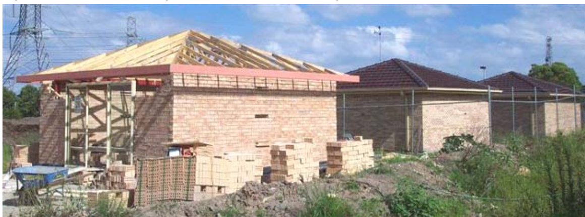
Figure 1. The three building modules for thermal testing
